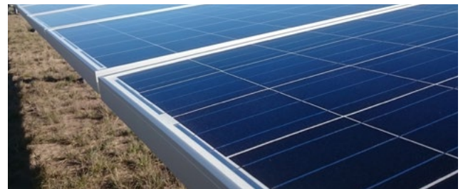
Single-axis tracking technology, seen here at Moree, will maximise the effectiveness of panels at Barcaldine Solar Farm
