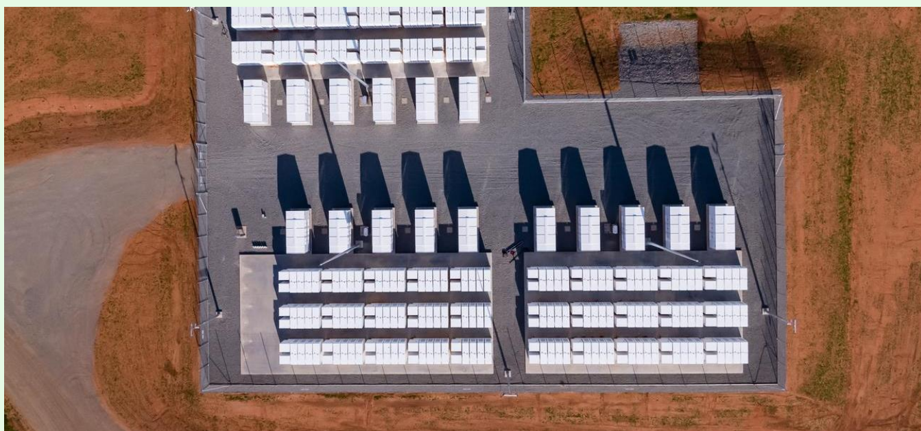
Figure 16: Li-ion batteries used on solar farm
