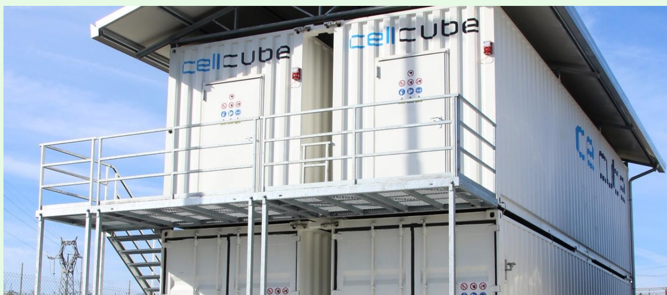
Figure 17: Vanadium redox flow battery, 400 kW/1.6MWh (image courtesy of Cellcube)
