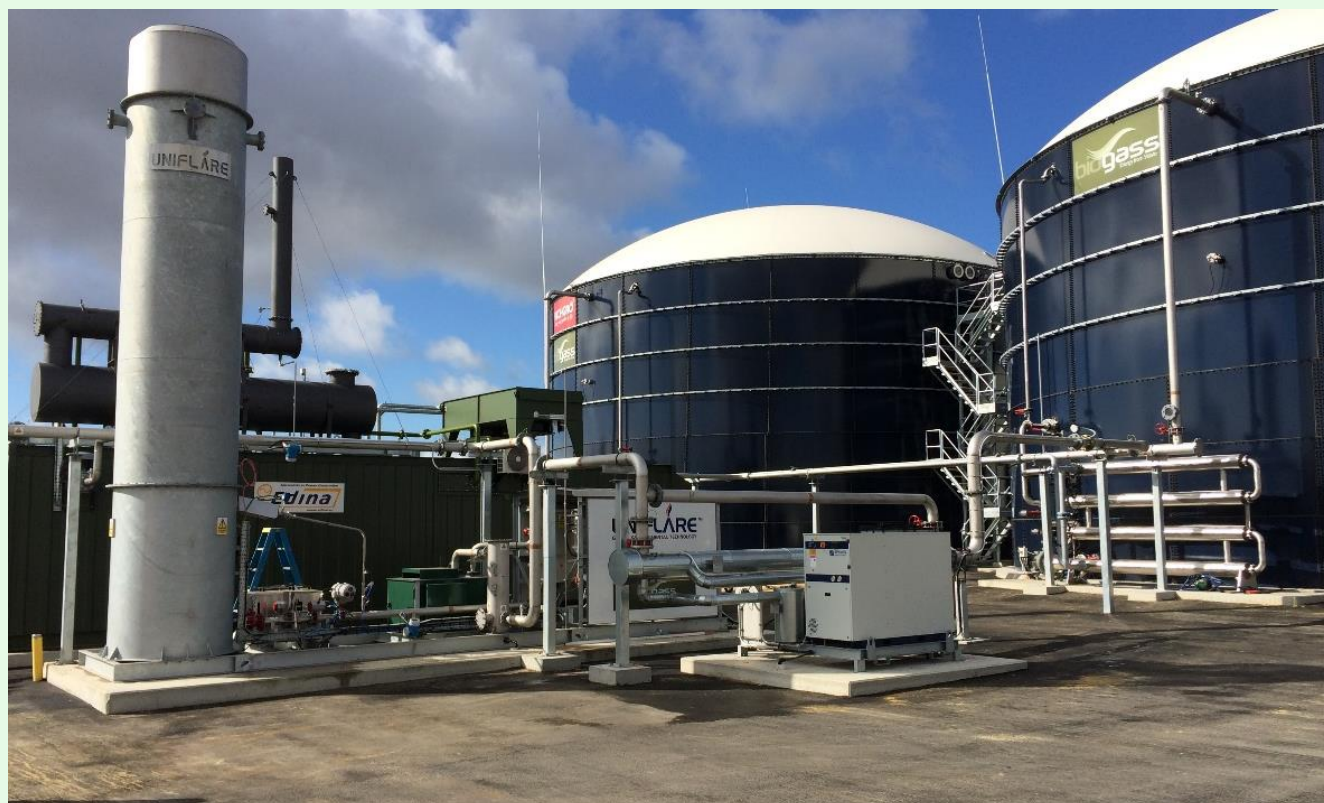
Figure 15: An anaerobic digestion facility at the Richgro site in Jandakot, WA (image courtesy of Delorean/Richgro)
